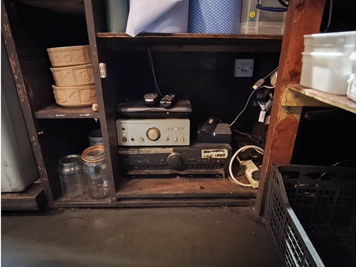
Figure 9: Amplifiers for the installed sound system are behind the ground floor bar
